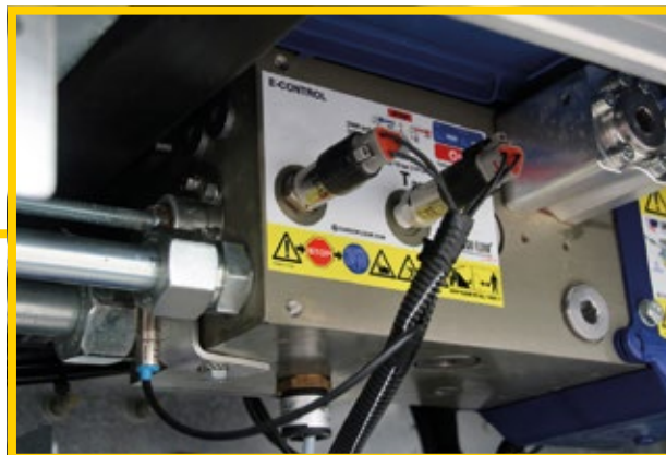
Oil pressure and temperature floor sensor
