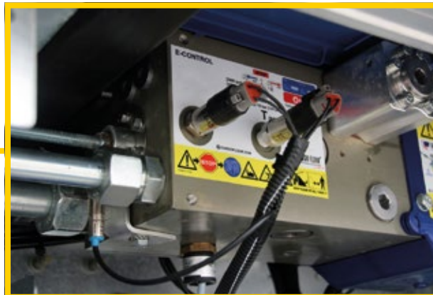
Oil pressure and temperature floor sensor
